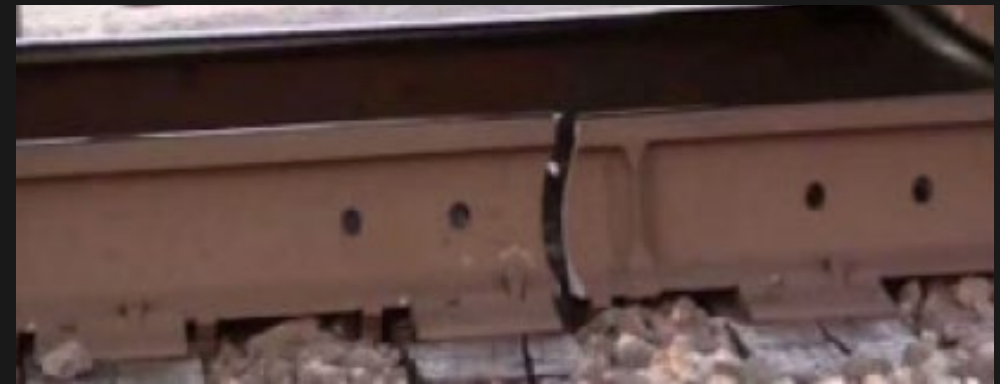
A broken rail due to extreme cold
