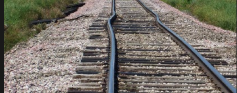
Track buckle due to extreme heat
