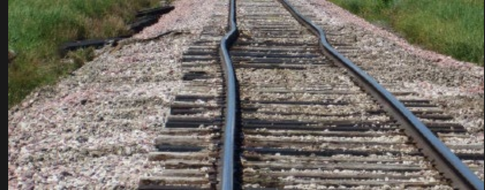
Track buckle due to extreme heat
