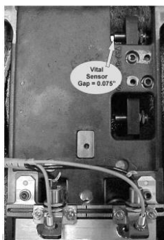
Figure 329(d)(2)-02: Lock Box Sensors
